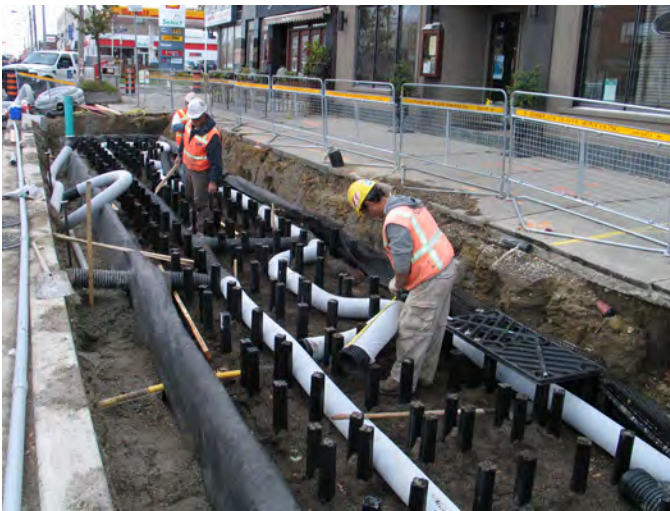
Streetscape Vaulted Paving Stormwater Capture and Irrigation System.
