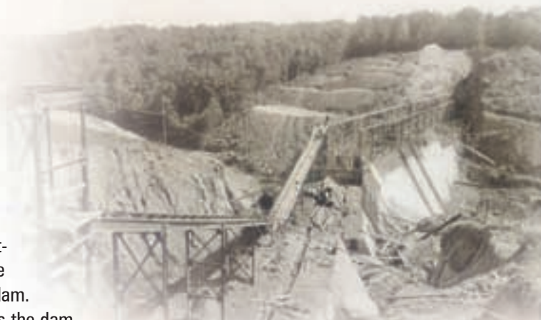
During construction, circa late 1920s. The Old Mill Stream Valley offered a natural basin, with high walls on three sides. Conveyor belts carried concrete to the dam.
