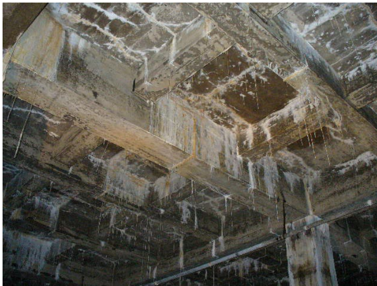
Deterioration of roof slab below paved areas in the west section Gredell & Associates, 13 July 2006
