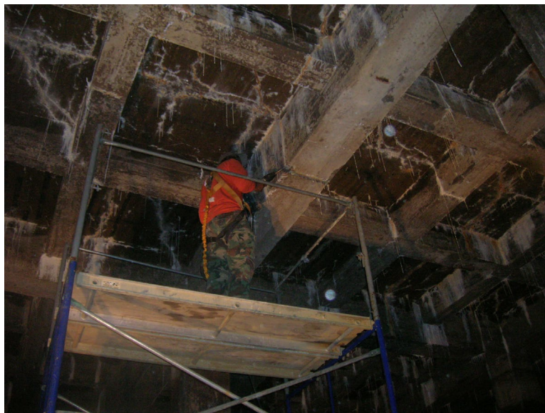
Probing the concrete girder with electric chipping tool to observe reinforcing steel Note: probe being made at construction joint Gredell & Associates, 31 August 2006
