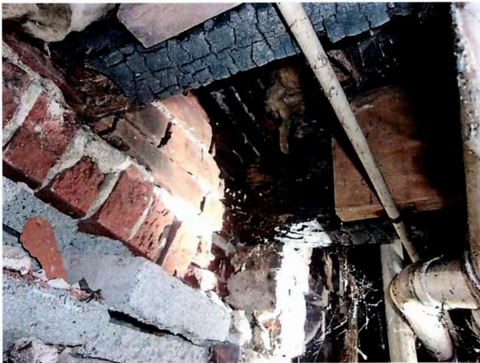
Photo 16 – Unsuitable bearing of framing at fire damage
