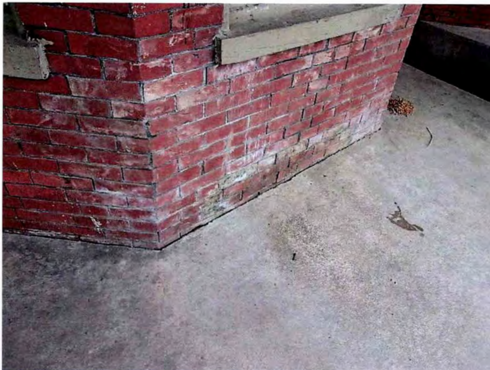
Photo 10 – Stains along front wall at 818 N. Adams Street
