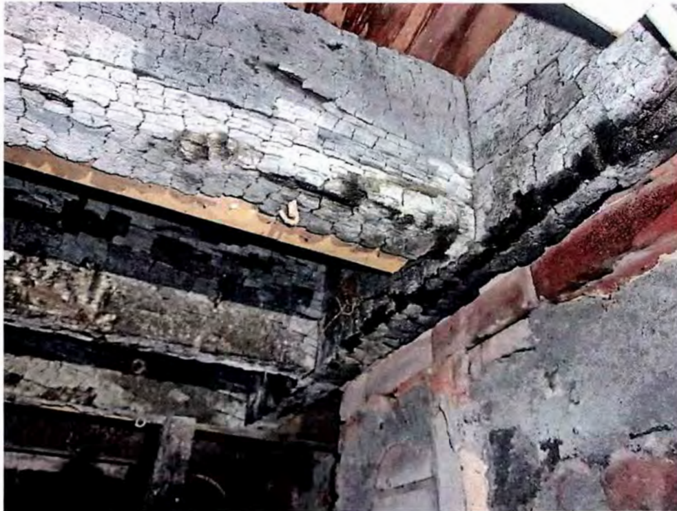
Photo 15 – Signs of fire damage at floor framing
