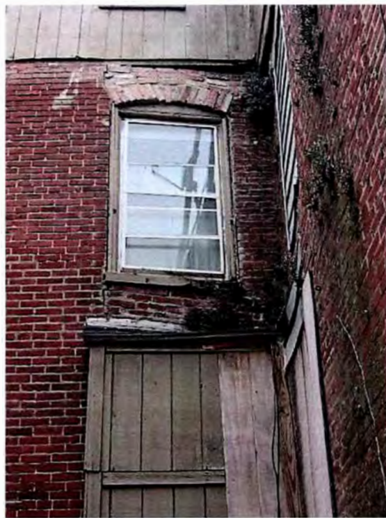
Photo 4 – Wall displacement along east face window
