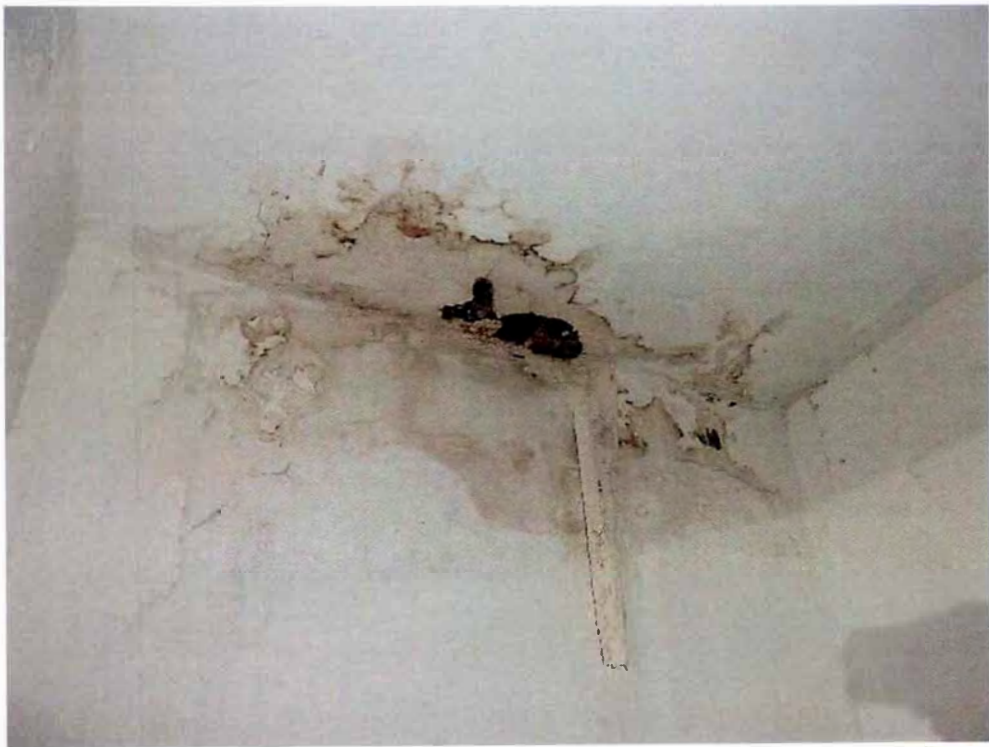
Photo 19 – Signs of rainwater infiltration at interior space
