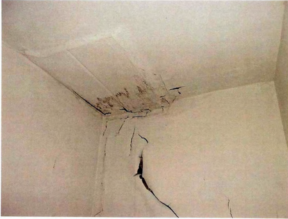
Photo 21 – Signs of rainwater infiltration at interior space
