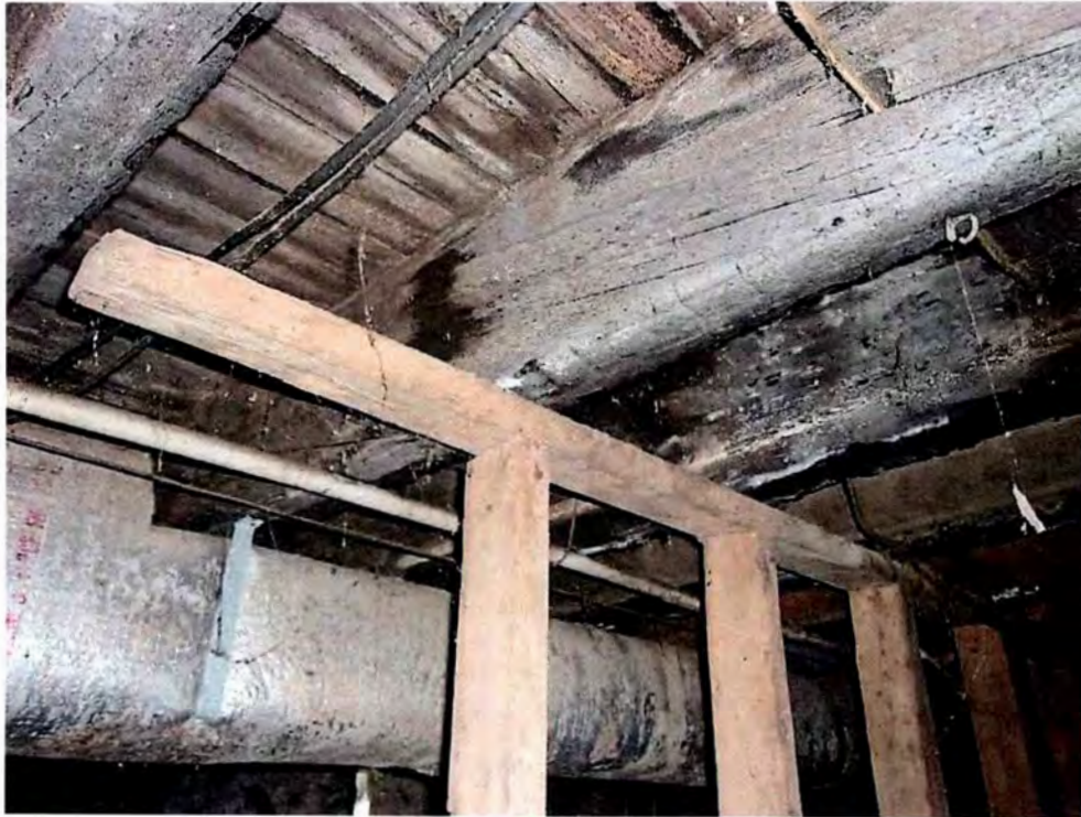
Photo 17 – Supplementary framing lacks positive connections to original framing
