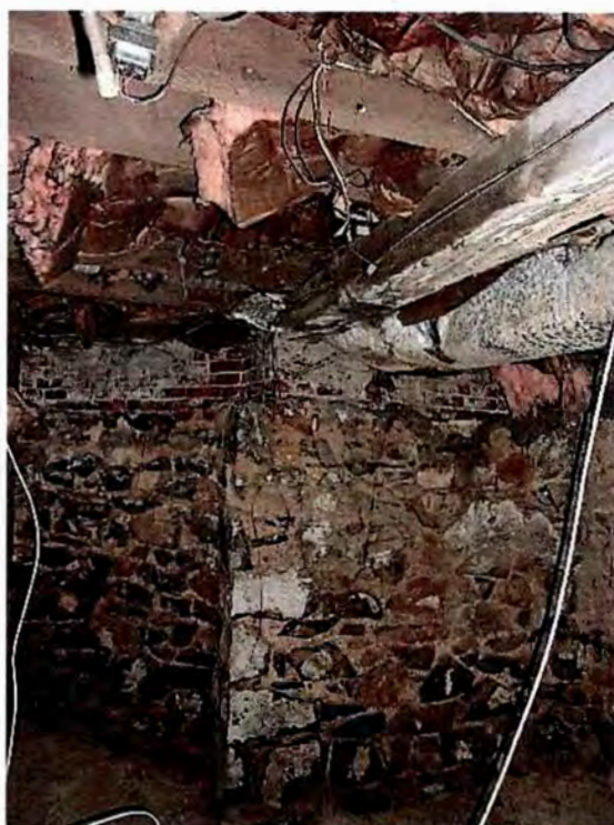
Photo 14 - Floor framing member lacks end support
