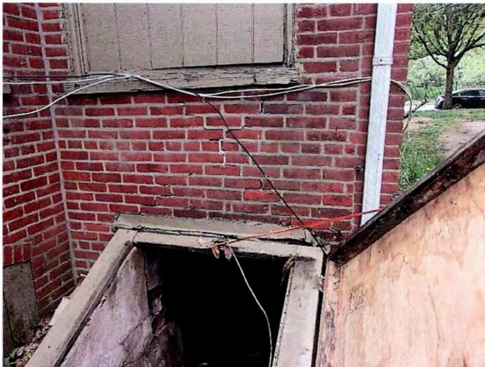
Photo 7 – Wall displacement/cracks above 820 N. Adams Street basement access
