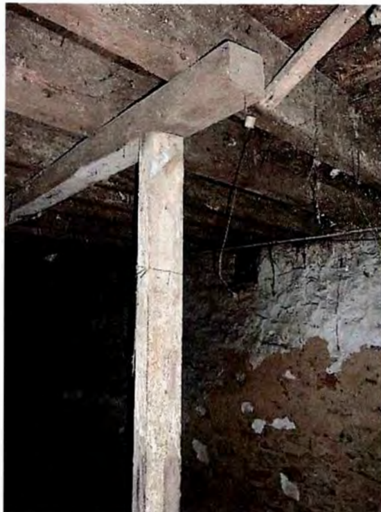
Photo 18 – Supplementary framing lacks positive connections to original framing
