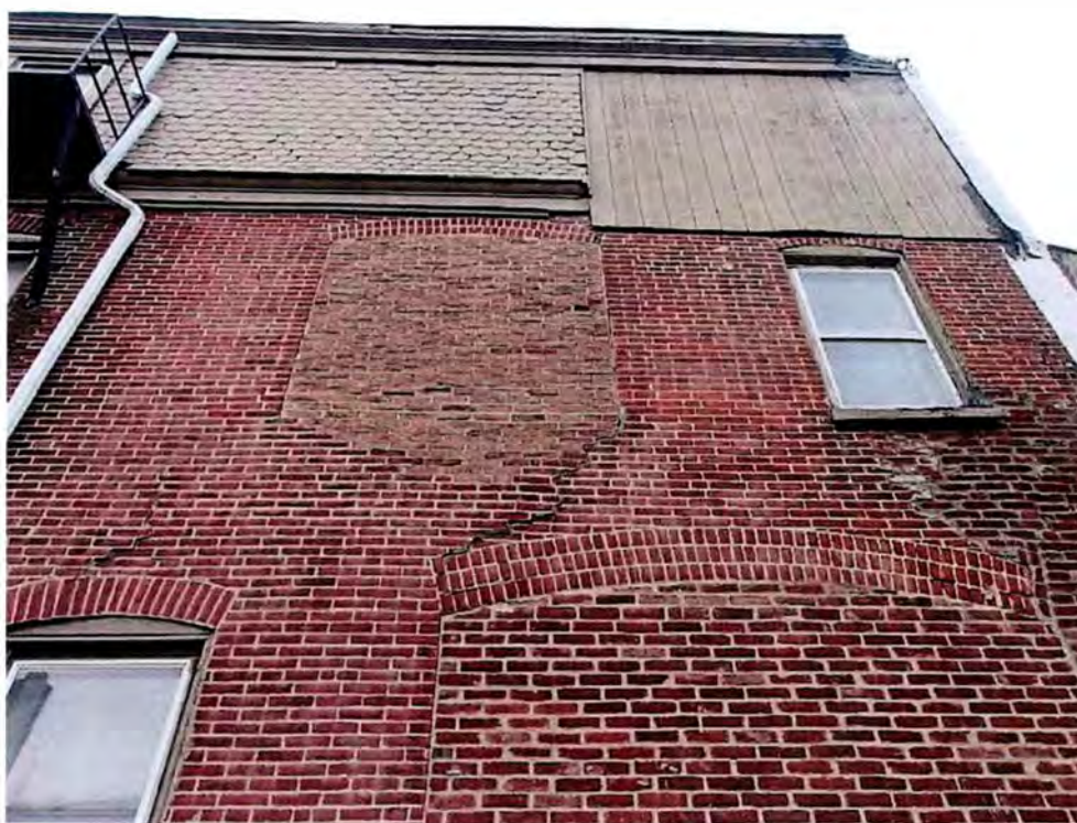
Photo 6 – Wall displacement/cracks along south face of 808/810 N. Adams Street
