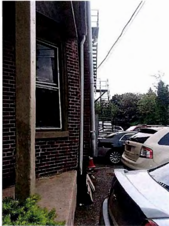
Photo 9 – Wall bowing along south face of 808/810 N. Adams Street
