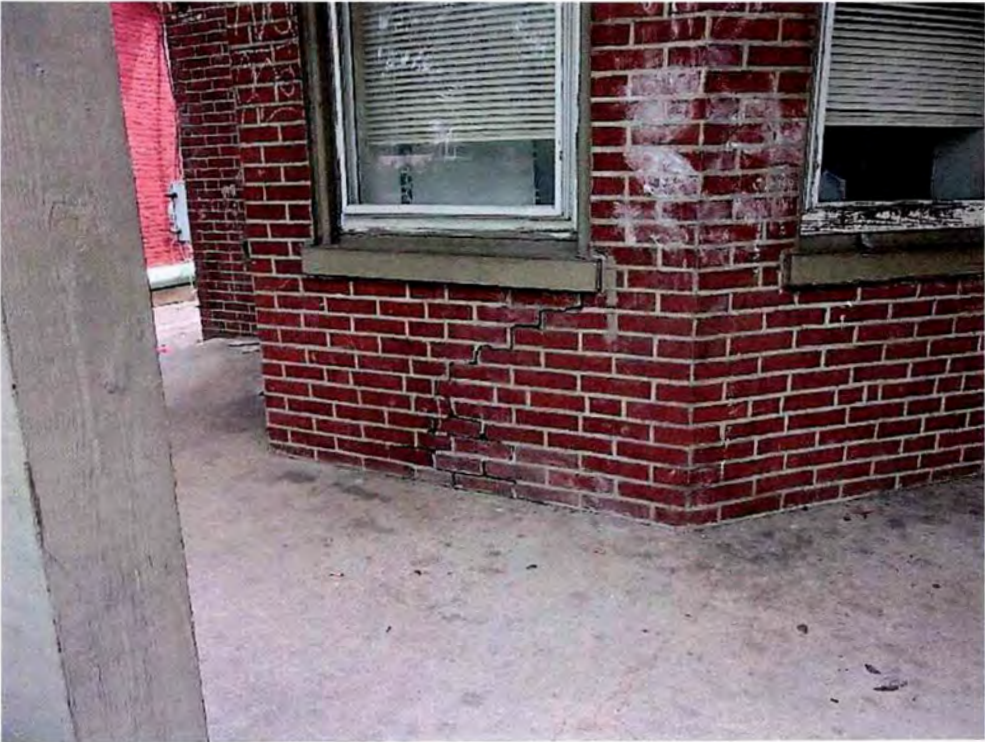
Photo 11 – Wall cracks/displacement along front wall at 820 N. Adams Street
