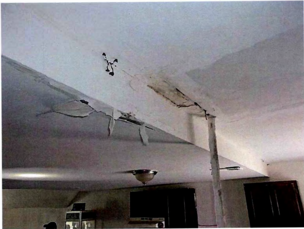
Photo 20 – Signs of rainwater infiltration at interior space
